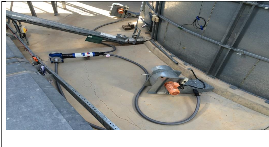
Fig. 5. A small fan (F370 – 0.37 kW) used during the first 5 days of fumigation to recirculate phosphine to give rapid uniform gas distribution in 1423 t wheat. See Figure 4.
